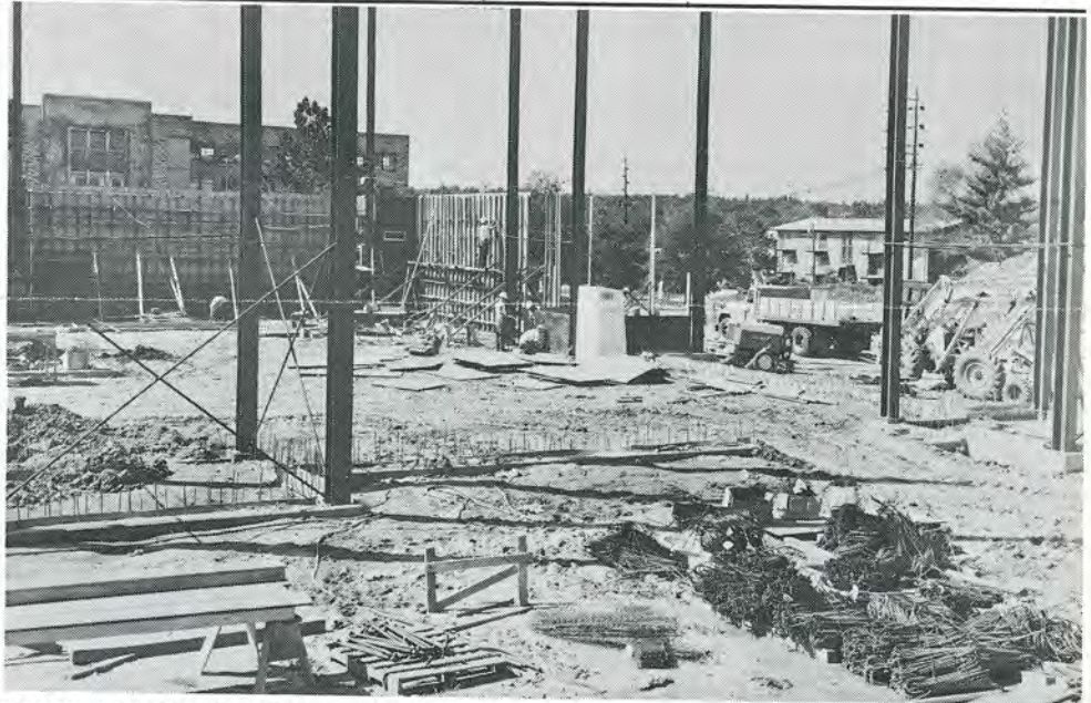
CONSTRUCTION PROGRESS on the new $2.8 million M. A. Durland Hall is on schedule on a building site west of Seaton Hall and north of Ahearn Fieldhouse. Durland Hall will house the chemical engineering and industrial engineering departments.
