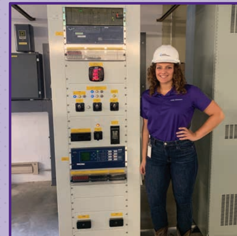
WORKING WITH THE RELAY SETTINGS GROUP, MACEY ELKINTON AT A SUBSTATION CONTROL PANEL IN STILLWELL THAT CONTAINS RELAYS FOR MONITORING TRANSMISSION LINES
