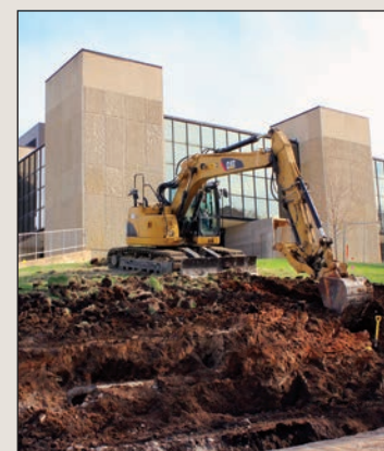
Above: Construction began in April on the 108,000-square-foot expansion to the engineering complex planned for completion in fall 2015.
